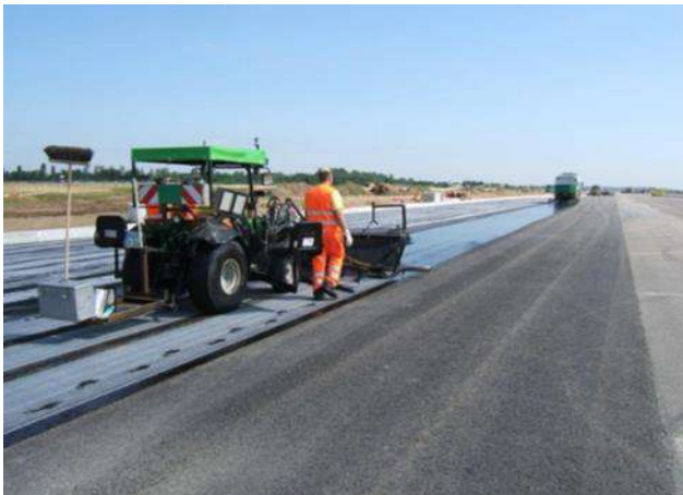
Tensar geogrids can strengthen weak subgrades and can control differential settlement, creating a mechanically stabilised layer for runways and taxiways.
